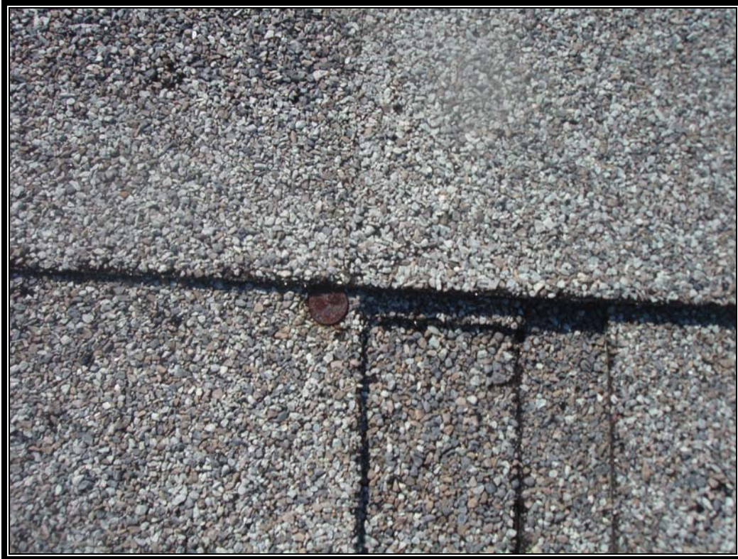
PHOTO #3: EXPOSED FASTENER – TYPICAL
