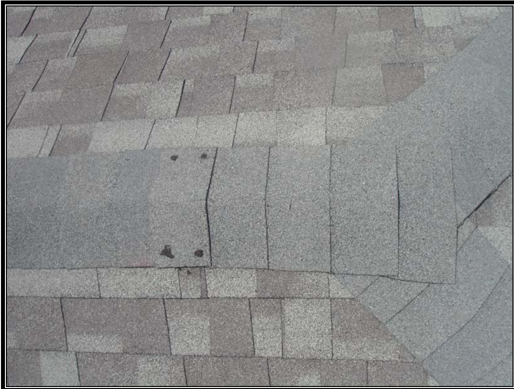
PHOTO #4: EXPOSED FASTENER - TYPICAL
